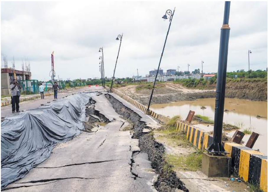
A large stretch of road caves in near the Bharat Ratna Shri Atal Bihari Vajpayee Ekana Cricket Stadium following continuous heavy rainfall, in Lucknow, Uttar Pradesh, Sunday.
