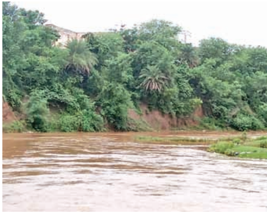
Soil erosion at the back side of District Hospital near Aagar river is posing threat to the District Hospital's foundation.
