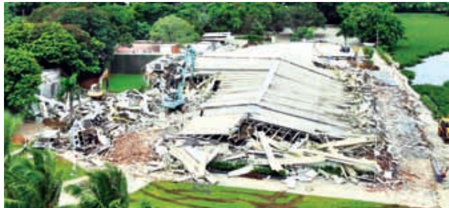
The N Convention, jointly owned by actor Nagarjuna, being demolished in Hyderabad. | Photo: PTI
