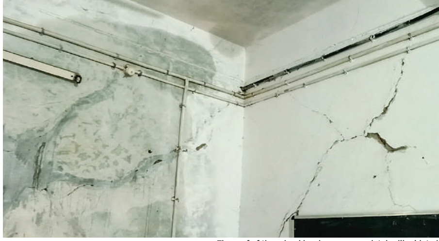
The roof of the school has become completely dilapidated.
