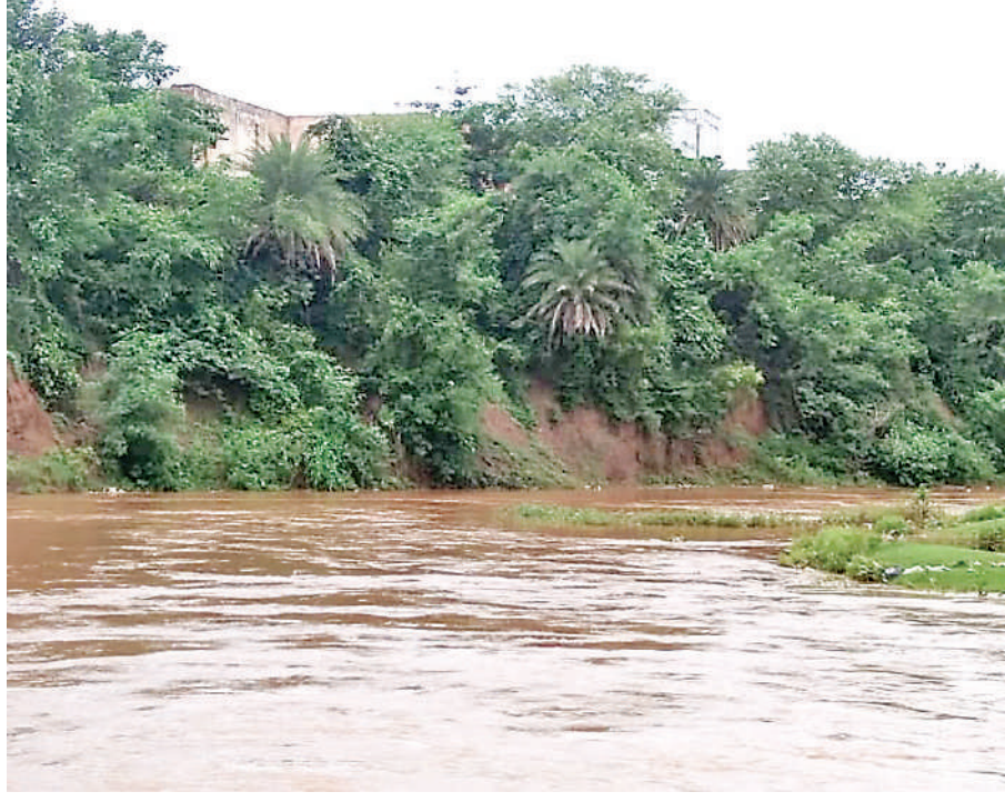
Soil erosion at the back side of District Hospital near Aagar river is posing threat to the District Hospital's foundation.
