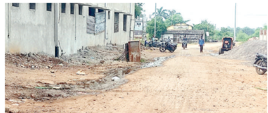
Contractor damages pipelines, causing water spill on road.
