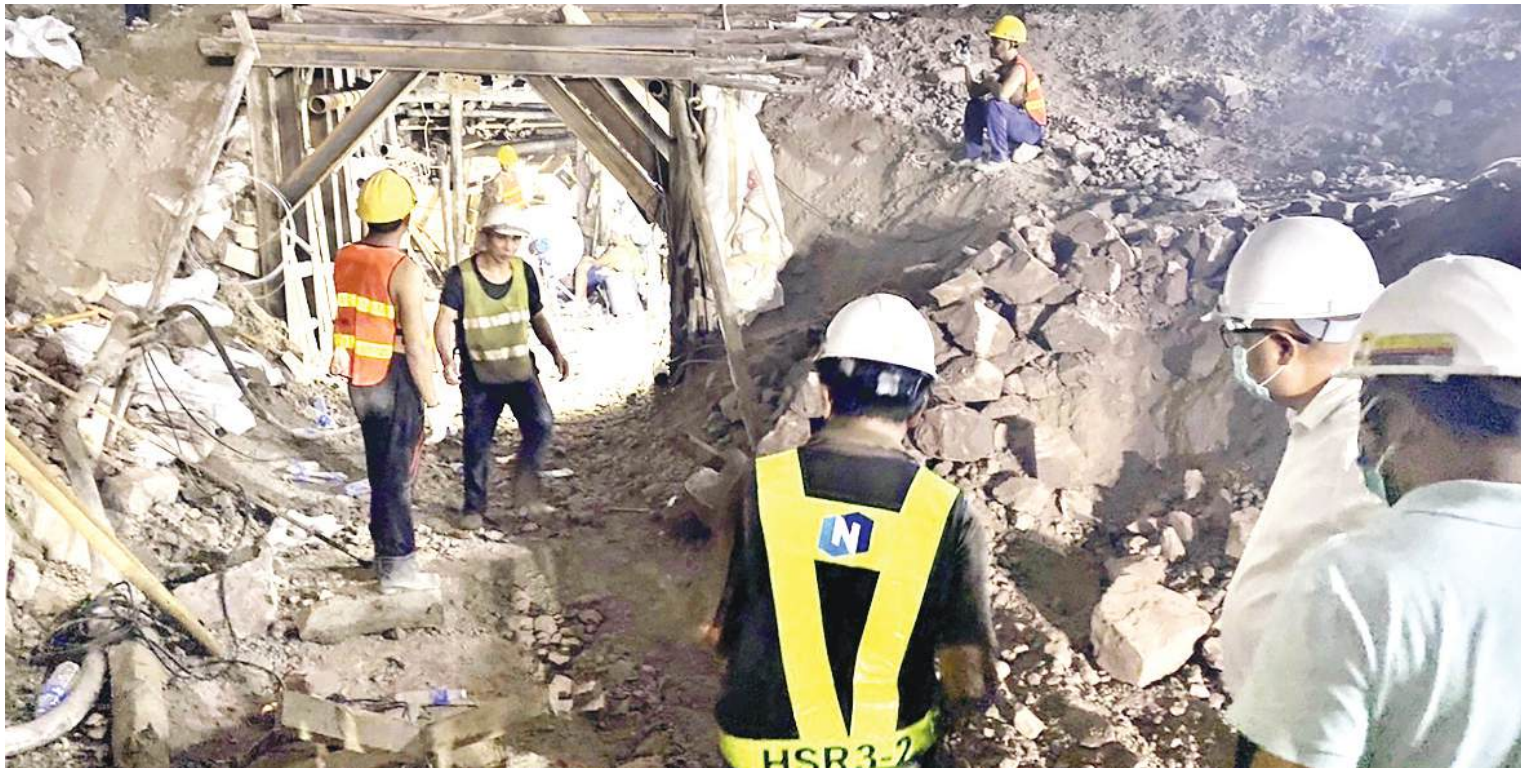
Rescuers work is on at Thai-Chinese high-speed railway construction site after collapse of a tunnel in Nakhon Ratchasima province. | Photo: PTI
