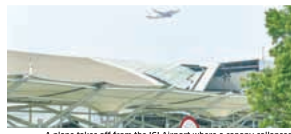
A plane takes off from the IGI Airport where a canopy collapsed.
