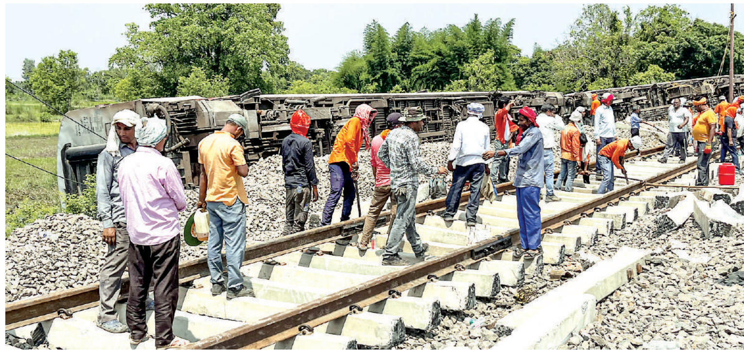
Technical staff and other workers during repair work on a railway track after the Chandigarh-Dibrugarh Express derailment in Gonda district on Friday. | Photo: PTI
