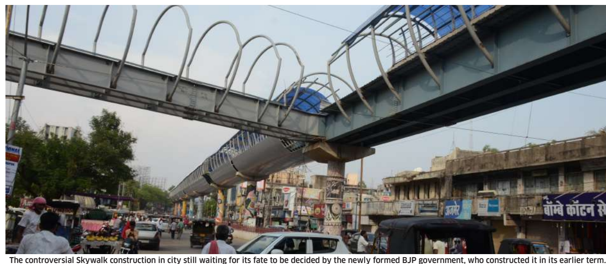
The controversial Skywalk construction in city still waiting for its fate to be decided by the newly formed BJP government, who constructed it in its earlier term.
