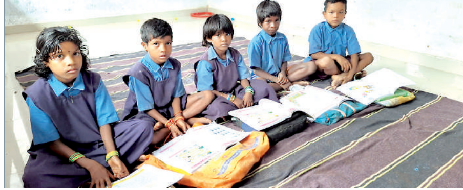
Since the school building has been renovated, there is no seepage in the classrooms now.
