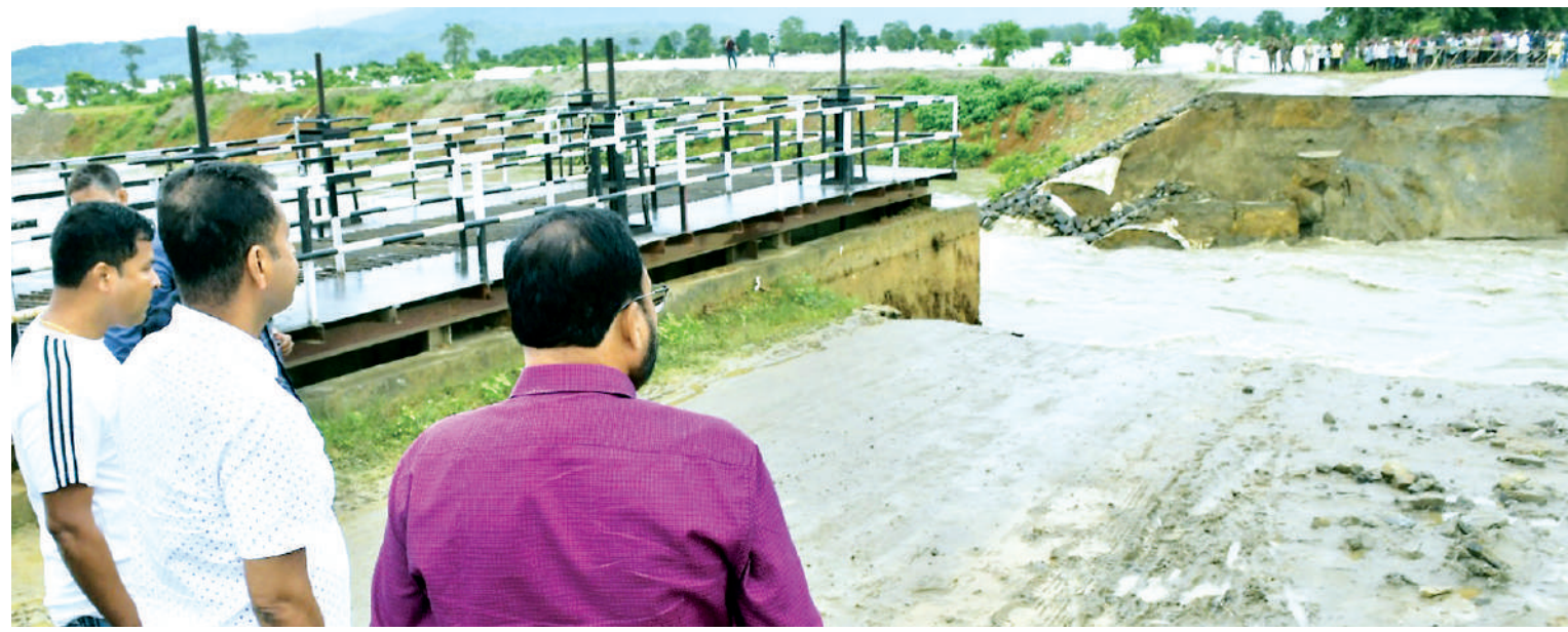
Assam minister Keshab Mahanta inspects an embankment that was damaged by flood water, at Hatimura in Nagaon district on Tuesday. PTI
