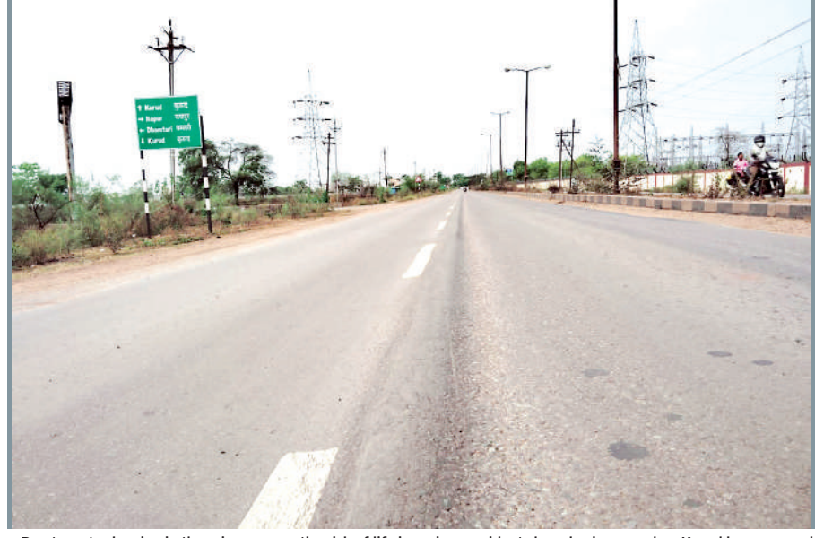
Due to water logging in the rainy season, the risk of life in serious accidents has also increased on Kurud by-pass road.
