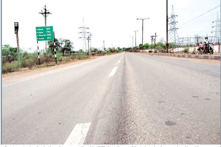
Due to water logging in the rainy season, the risk of life in serious accidents has also increased on Kurud by-pass road.
