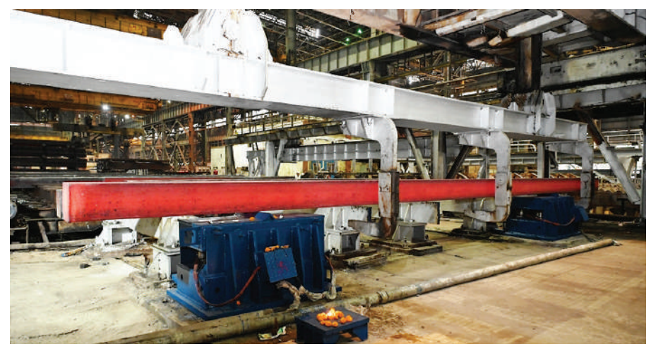
Bloom weighing system installed in CV 1 caster.
