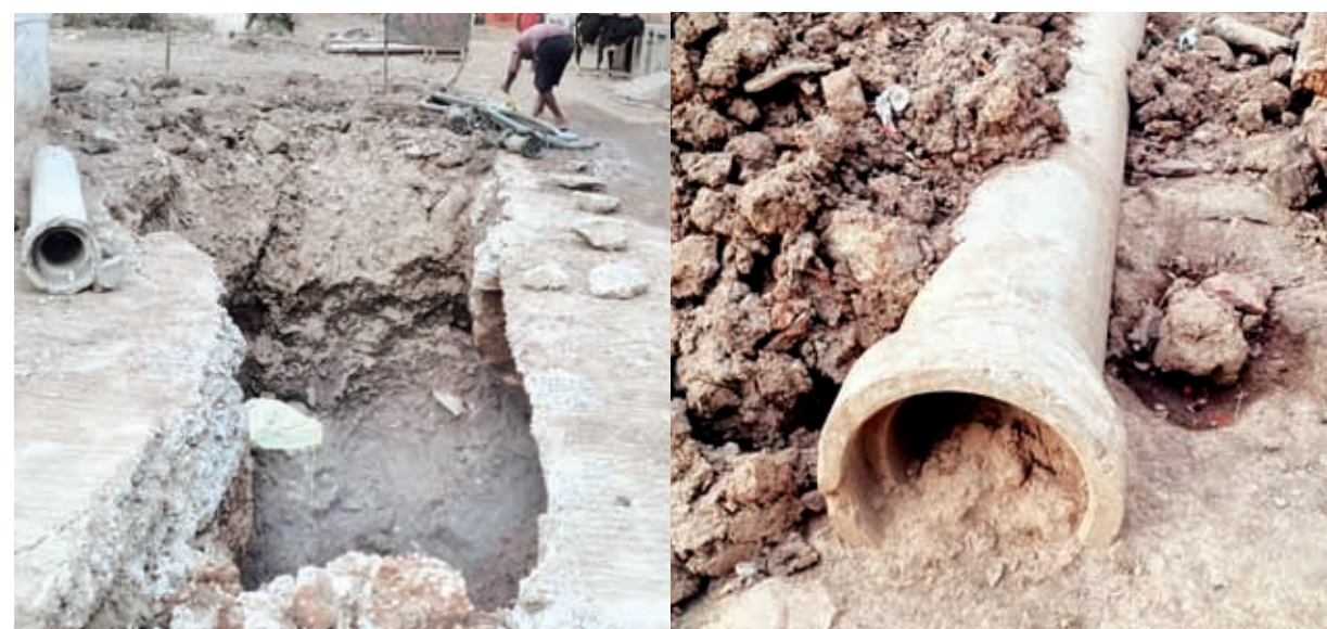
Urban Administration and Development Department is constructing a sewerage treatment plant near Shivnath river.
