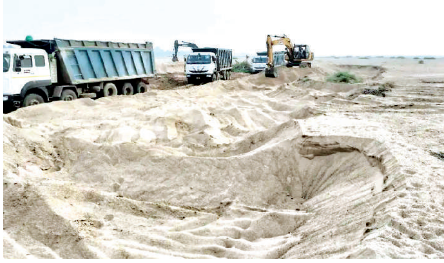
Illegal mining by sand mafias in Gram Lachkera is going at a rampant pace, under the guise of new methods and rules.
