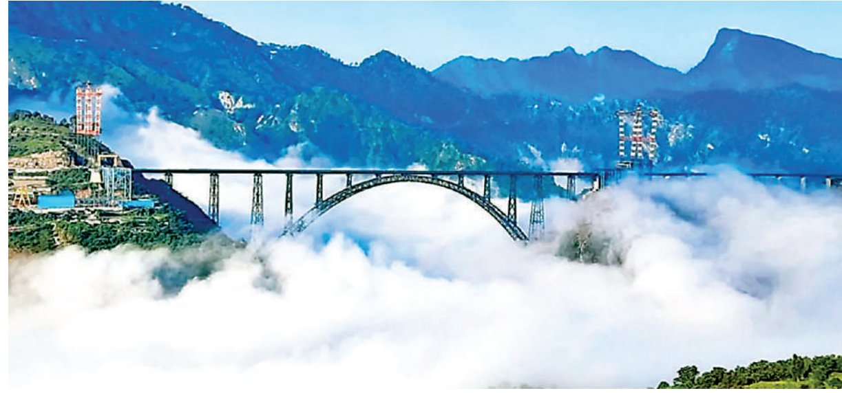
Railway bridge being constructed 359 metres above the bed of Chenab in J&K.
