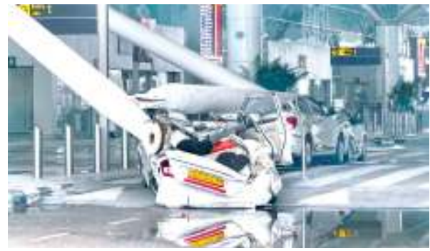
Roof of a canopy collapsed at Delhi airport. PTI
