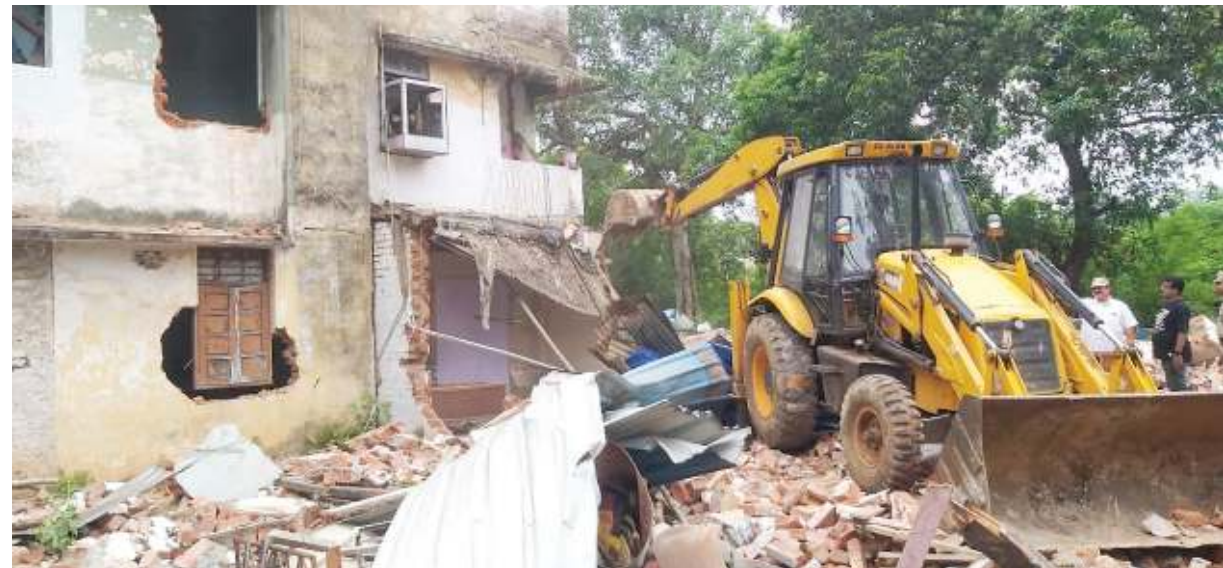
The administration took bulldozer action against a notorious offender.
