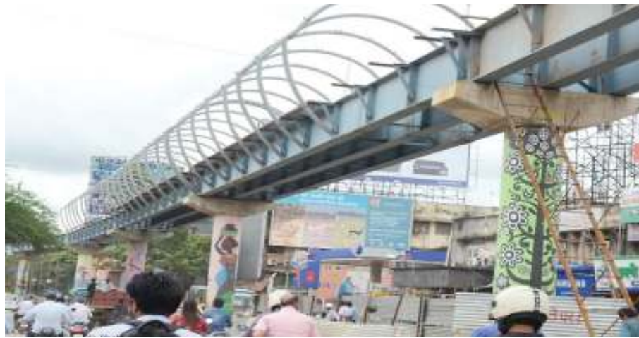
Sky Walk project in depilated condition.
