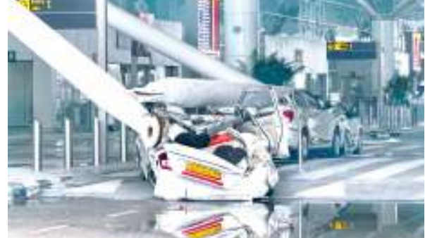
Roof of a canopy collapsed at Delhi airport. PTI
