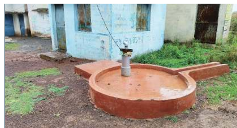
Drinking water is being supplied by installing a power pump in Pirchatola.
