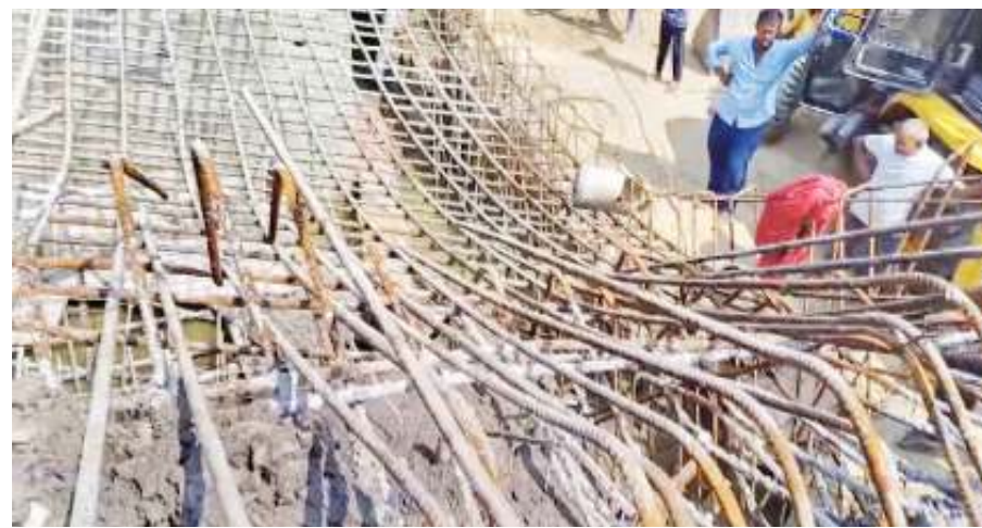
A portion of the under-construction bridge after it collapsed.
