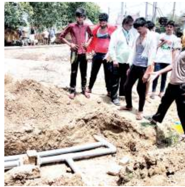
Workers are fixing the line to get water supply from one of the sources.
