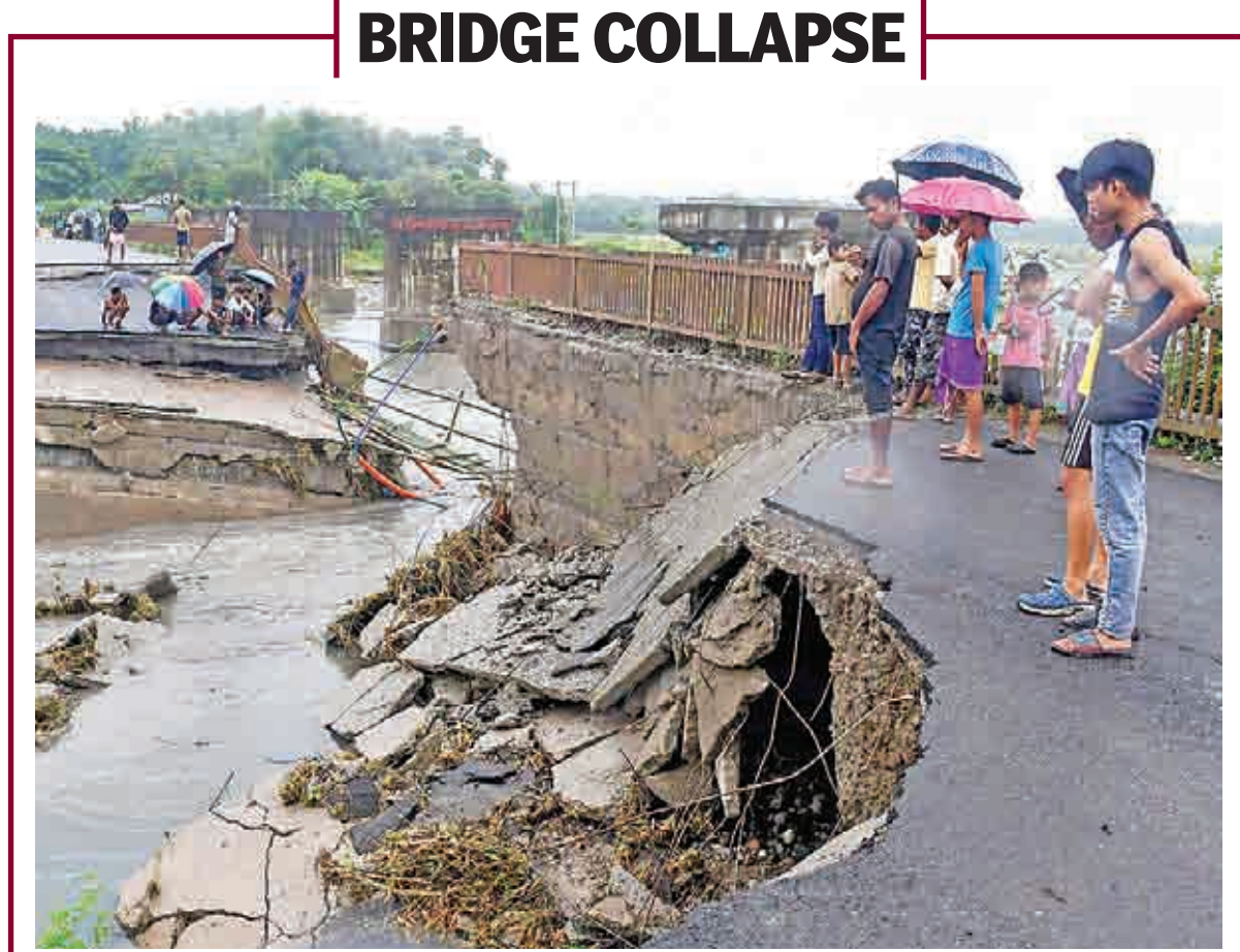
Villagers near the collapsed bridge over the Daranga River at flood-hit Kumrikata in Baksa district, Friday.
