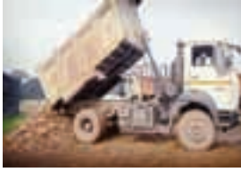
BHILAI: Acting on the directives of Collector Abhijeet Singh, road repair work has commenced at the Selud and Arasnara paddy procurement centres in Durg district.
